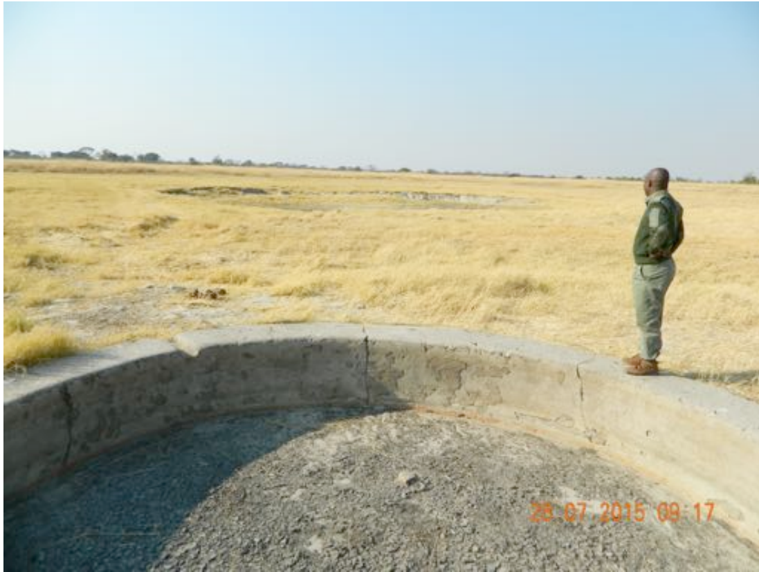
Kazuma – Corner Pan on the edge of the Depression – many years since pumped.
