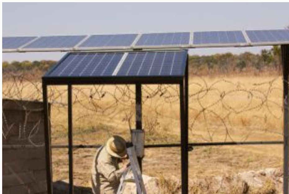
Wiring up the two extra panels on No 3 – noticeable extra flow straight away
